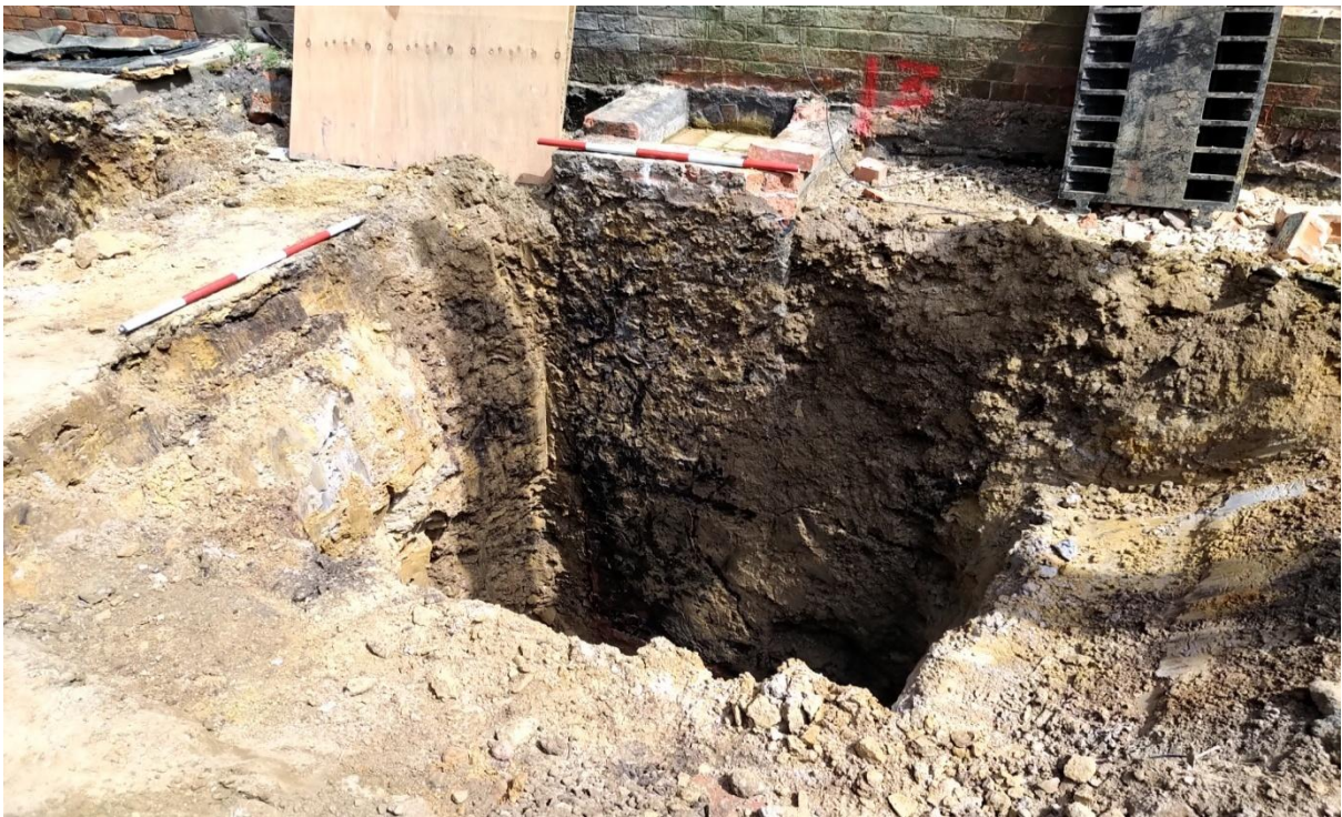
Plate 24: Providing more detailed overlook on foundation pads excavated in north-western part of the site adjacently to existing building to the east. Looking east, one metre scales.
