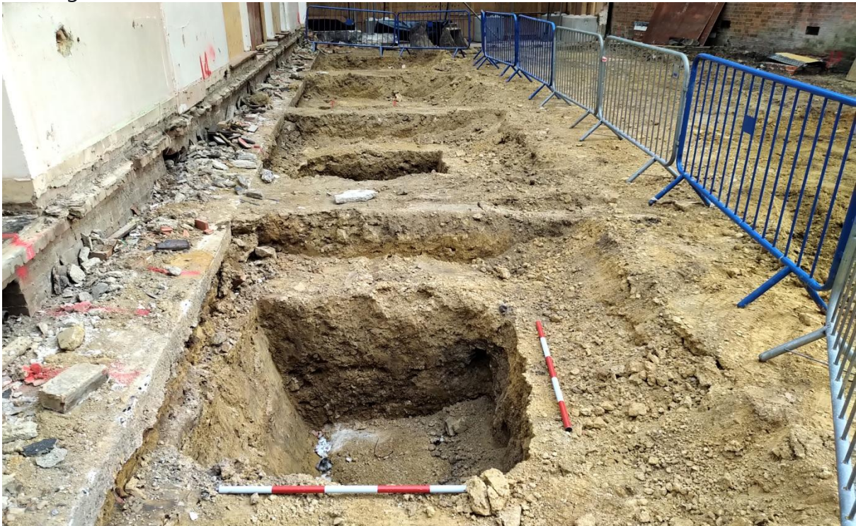
Plate 18: Showing excavated foundation pads in north-western part of the site beneath demolished Lending library. Looking north; two one-metre scales.
