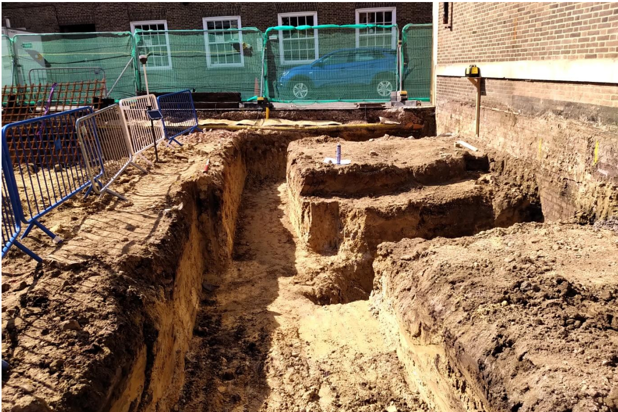
Plate 12: Showing foundations in south-western part of the site, adjacent to existing building. Looking south, one metre scale.
