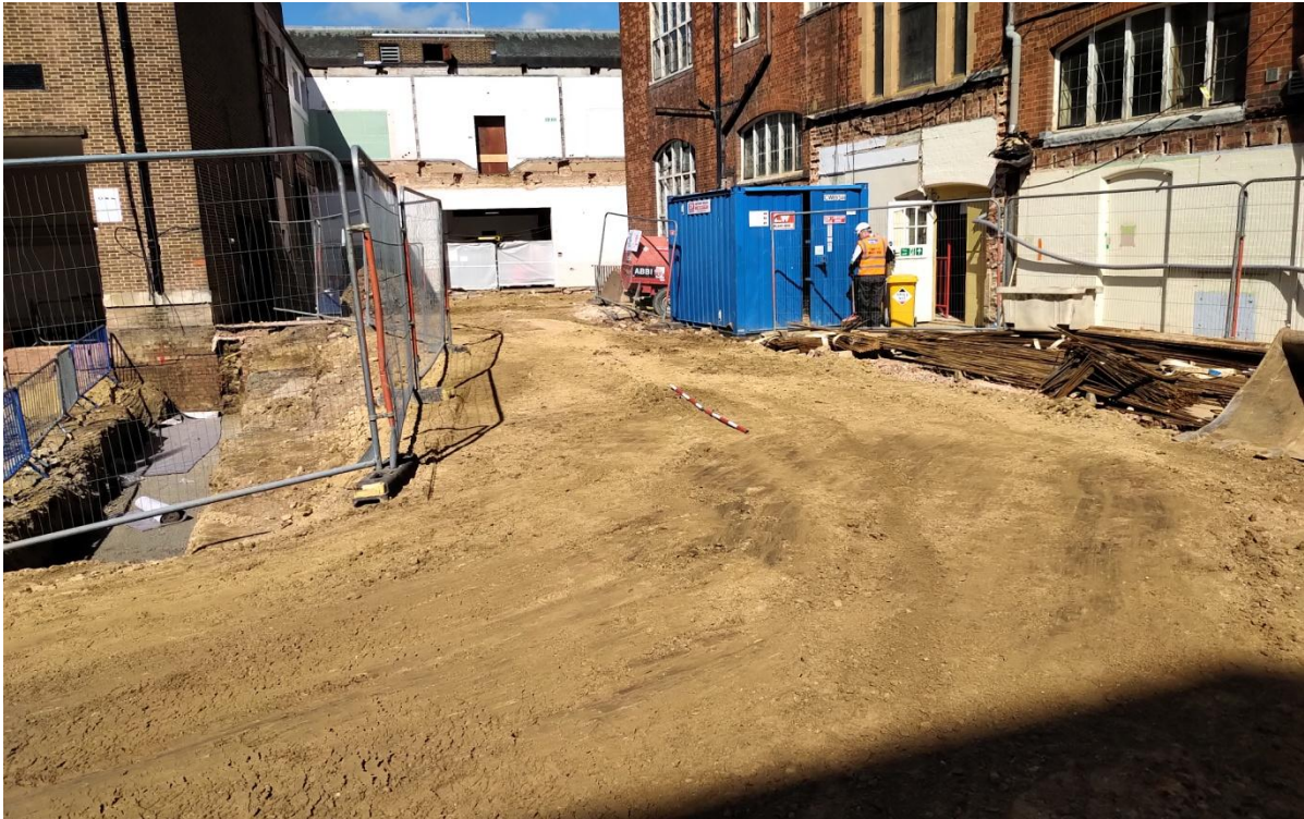
Plate 17: Showing exposed ground in northern part of the site prior to excavation. Looking west with two metre scale.
