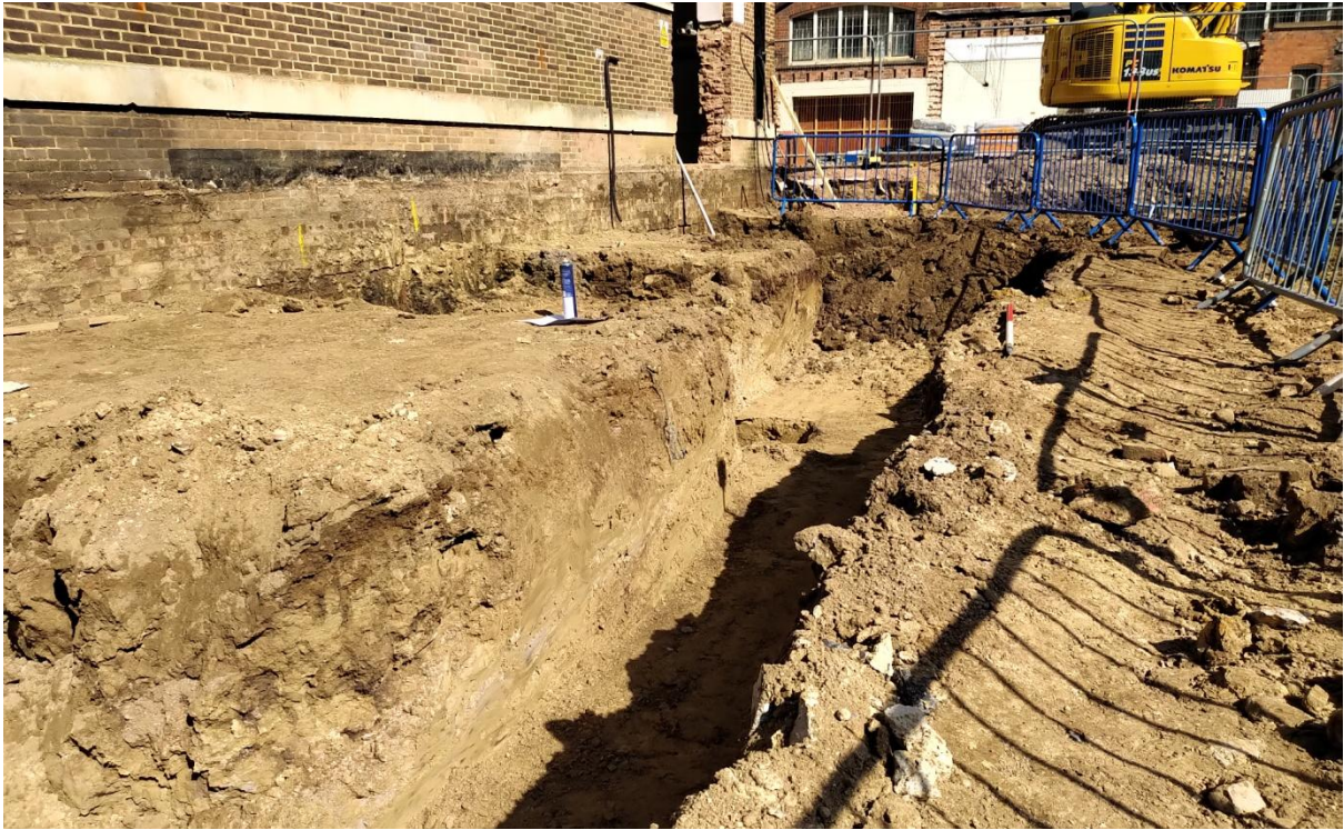
Plate 13: Showing foundations in south-western part of the site, adjacent to existing building. Looking north, one metre scale.
