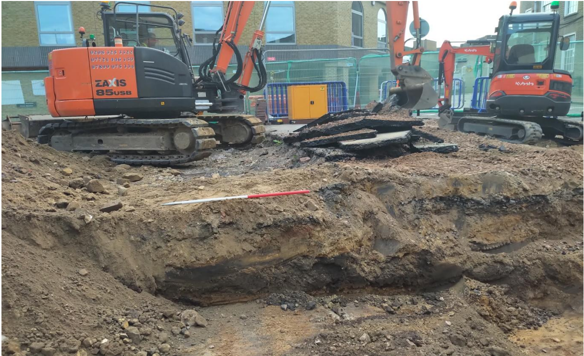
Plate 5: Showing section through reduced made-up ground in southern part of the site. Looking east with 1 metre scale.
