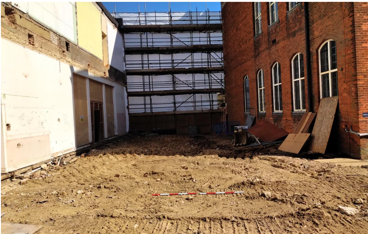
Plate 16: Showing exposed ground beneath demolished Lending Library (north-western part of the site) prior to commencement of excavations. Looking north with two-metre scale.
