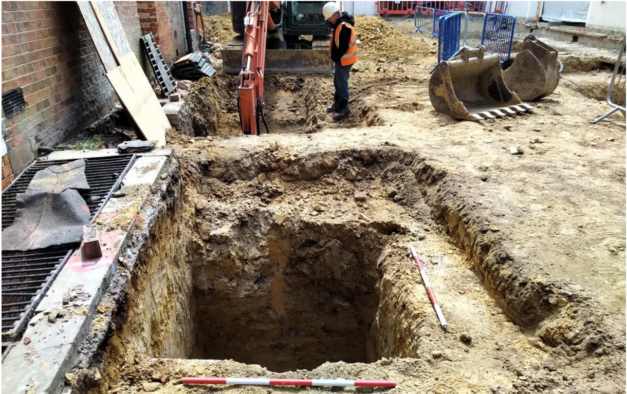
Plate 23: Showing on-going excavation of foundation pads in north-western part of the site adjacently to existing building to the east. Looking south, one metre scales.
