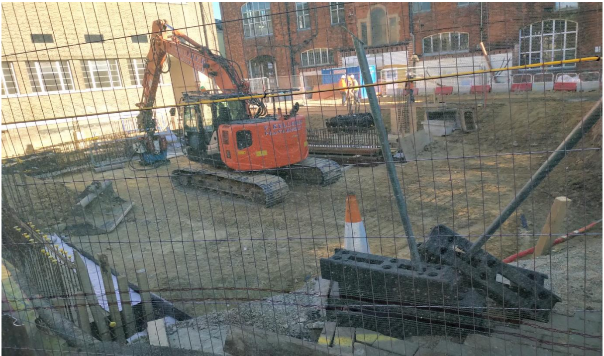
Plate 26: An overlook onto southern part of the site as construction works progresses. Looking northwest.
