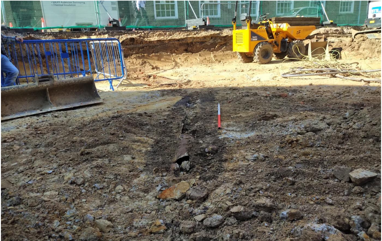
Plate 9: Showing an old culvert revealed in southern part of the site. Looking southwest with one metre scale.
