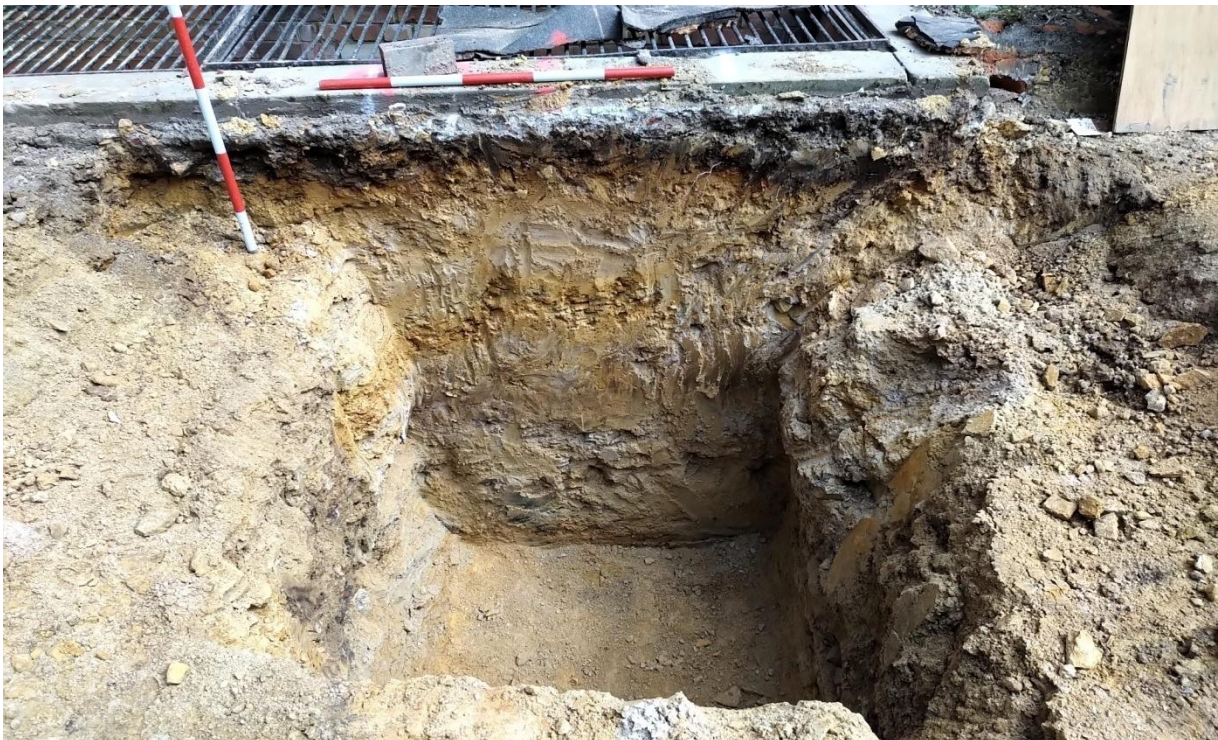
Plate 22: Providing more detailed overlook on foundation pads excavated in north-western part of the site adjacently to existing building to the east. Looking east, one metre scales.
