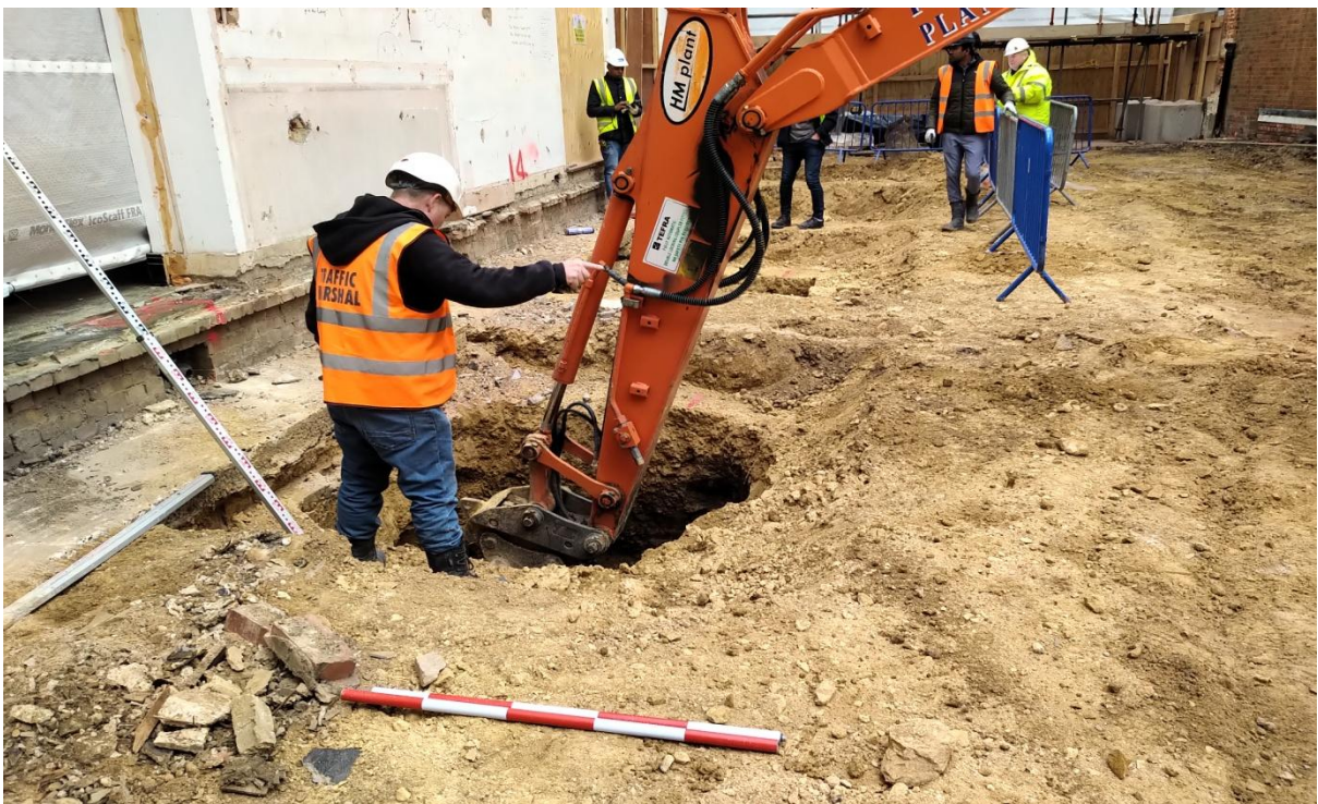
Plate 20: Showing further deepening of foundation pads in north-western part of the site with one metre scales.
