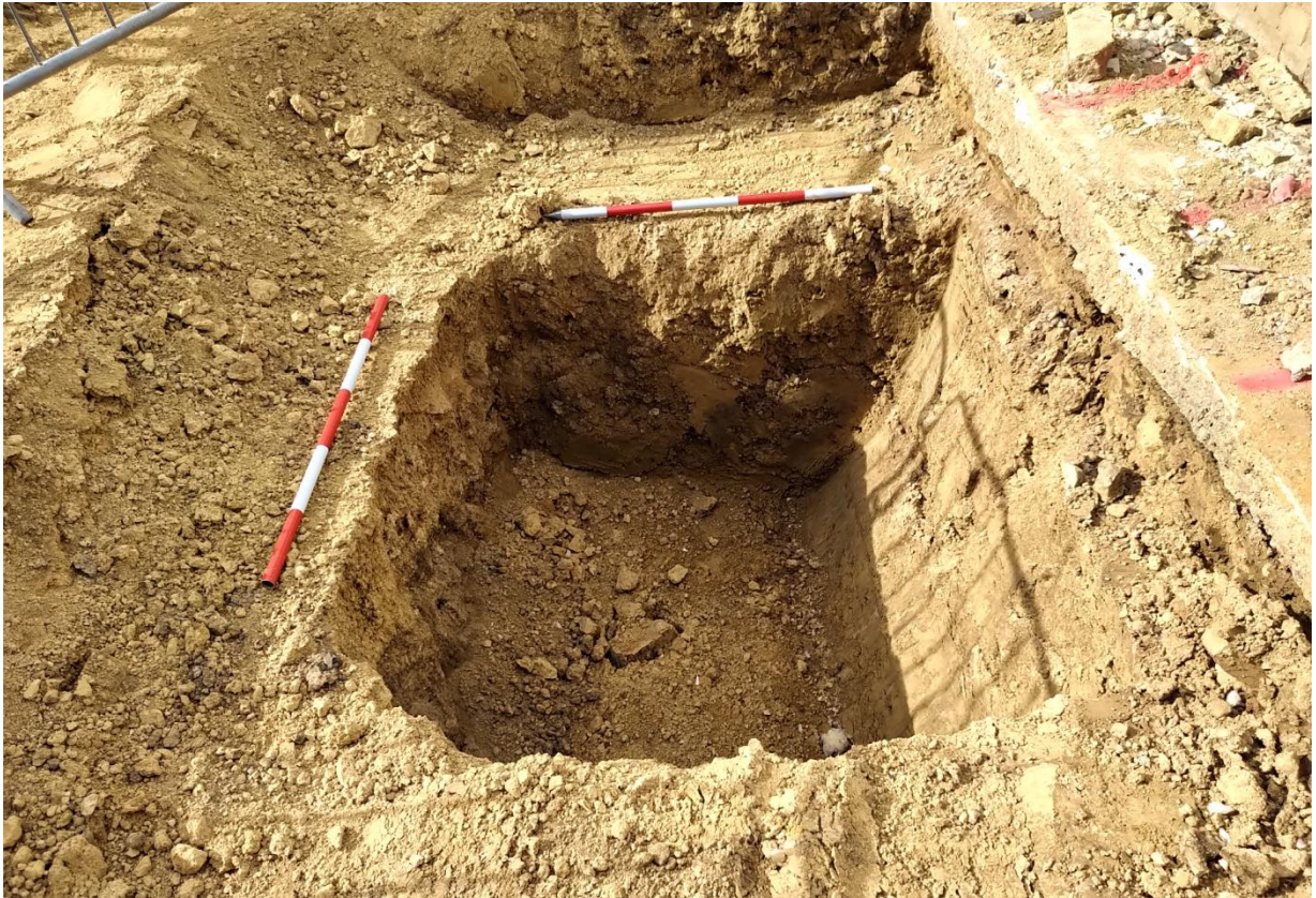
Plate 19: Providing more detailed overlook on excavated foundation pad in north-western part of the site. Two one metre scales.
