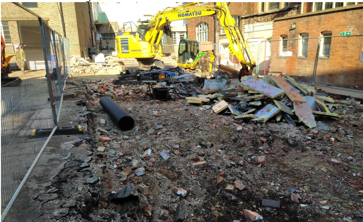
Plate 2: Showing northern part of the site. Demolition of Lending Library in the background and removal of demolished material in foreground. Looking west.
